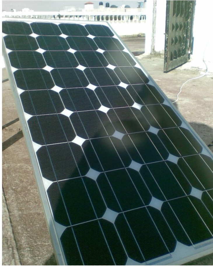
Figure 5.3: Mounted PV Module on roof building
