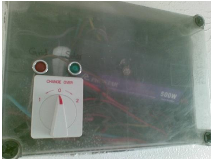
Figure 5.6: 500W Inverter with changeover switch between grid network and solar system
